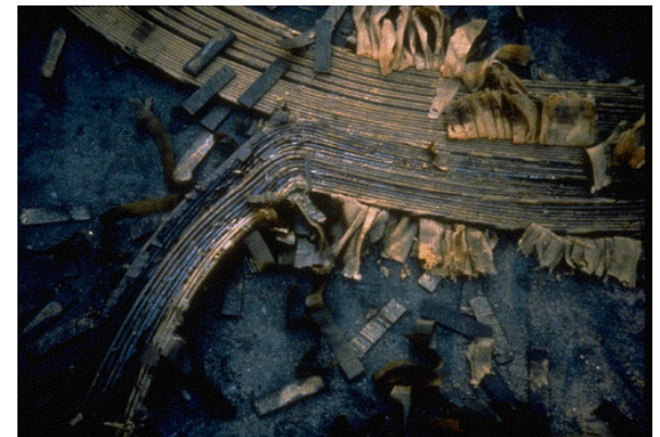
Melted 500kV transformer coil from EM induced flux creating a hot spot
